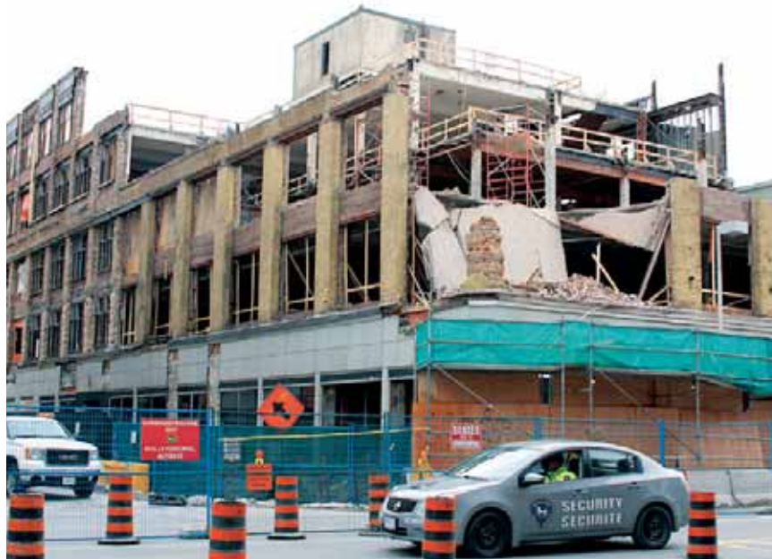
A security guard sits in a car outside the Ogilvy building. A section of the structure's facade collapsed on Saturday.
